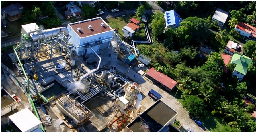
Fig 2: Bouillante power plant in Guadeloupe
